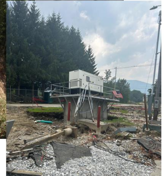
Ludlow, VT WWTP, floods July 2023
