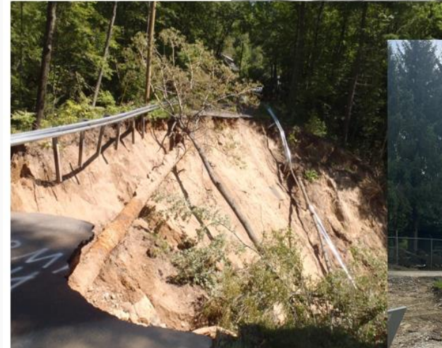
Bristol, CT WTP, floods Sept. 2011
